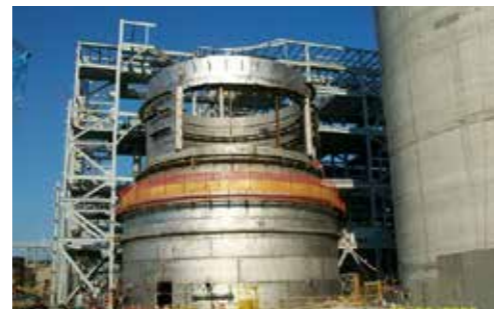
Scrubber for Reliant Project for Keystone USA
