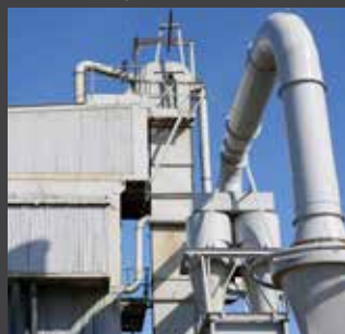
Dust and fly ash extraction pipes ▼
