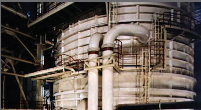
A scrubber in Flue Gas Desulfurization system made of 625 cladding ▲
