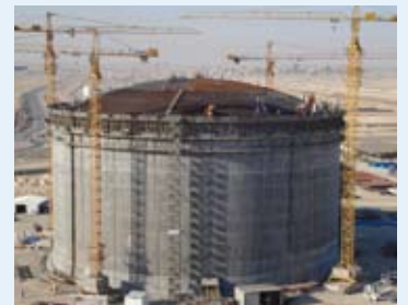
LNG tank under construction for RasGas co Ltd by MHI in Qatar
