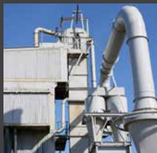
Dust and fly ash extraction pipes ▼
